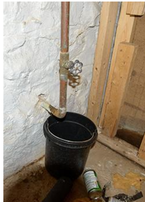
Figure 3: Copper service line
