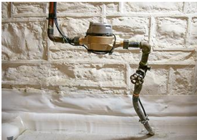
Figure 1: Lead service line
